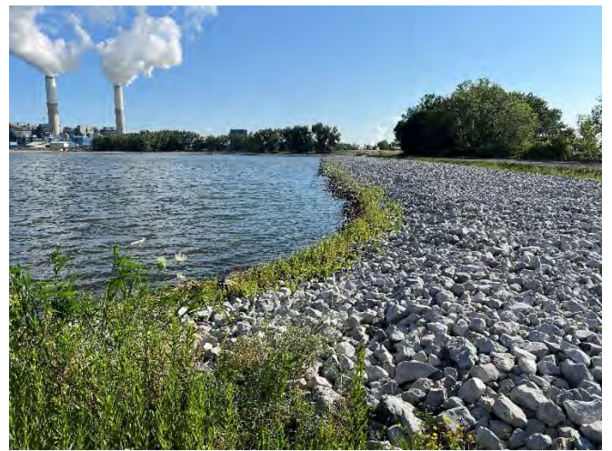
Photo 8: East internal slope of impoundment, view from south separation berm at southeast corner of impoundment. Riprap cover, typical of east and north slopes. Some vegetation growth near water line.
