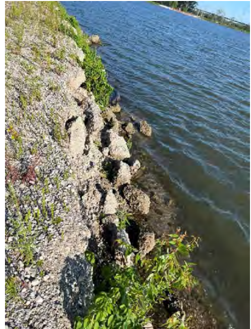
Photo 6: Sloughing and erosion of south separation berm (impoundment side).
