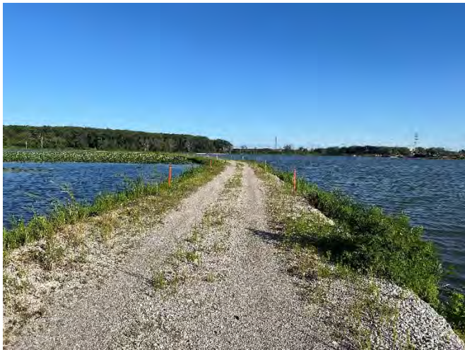
Photo 7: South separation berm, looking west. Vegetation growth on both sides. Roadway in fair condition, however closed to vehicular traffic due to north (impoundment side) slope sloughing as seen in photo 6.
