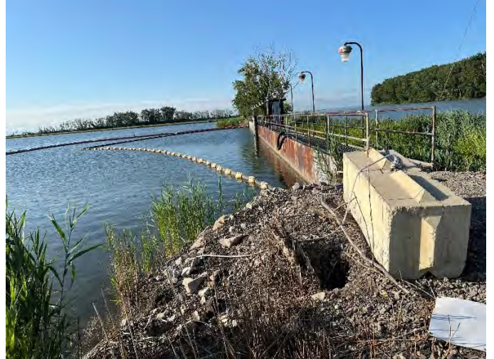
Photo 2: View of upstream side of principal spillway structure from north. Small sinkhole visible in foreground. A few similar sinkholes behind concrete bin block, not visible.
