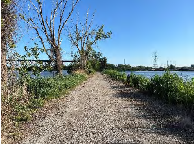
Photo 1: Western perimeter dike, looking north. Gravel road in satisfactory condition. Heavy vegetation visible on both slopes, with large/woody vegetation on downstream/west slope.
