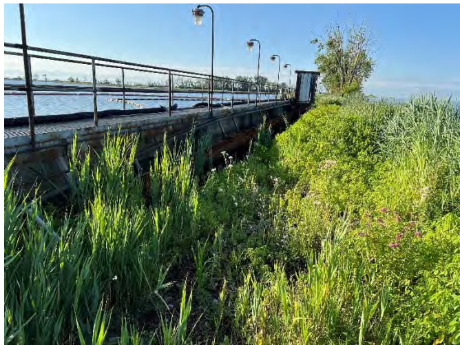
Photo 3: View of downstream side of principal spillway structure from north. Riprap outlet channel overgrown with vegetation.
