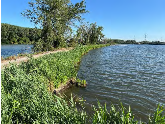
Photo 5: Impoundment side of western perimeter dike, looking north. Photo taken from separation berm at southwest corner of impoundment.
