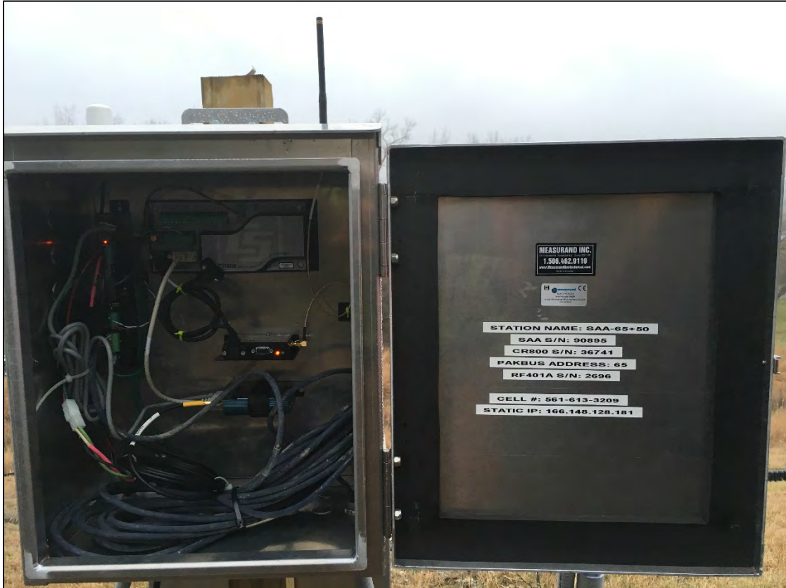
Figure 6. Inclinator SAA-65+50 EarthStation Interior
