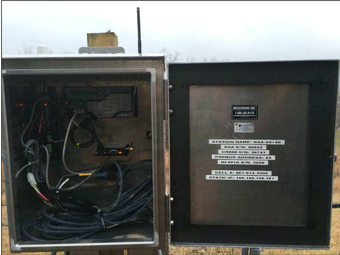
Figure 6. Inclinator SAA-65+50 Earthstation Interior
